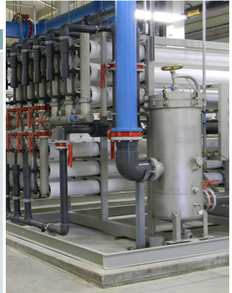
Typical Reverse Osmosis Skid
