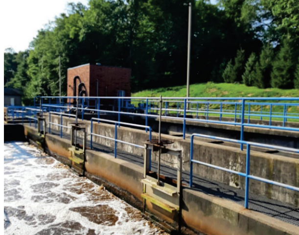
Existing Aeration Tanks
