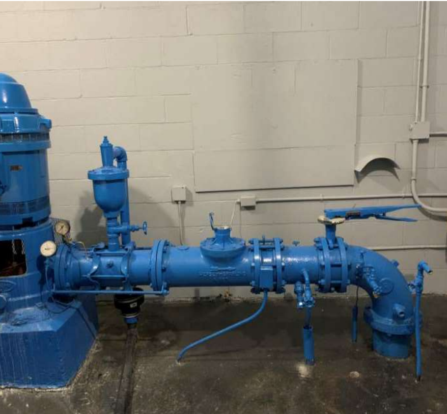
Interior of Wellhouse No. 6
