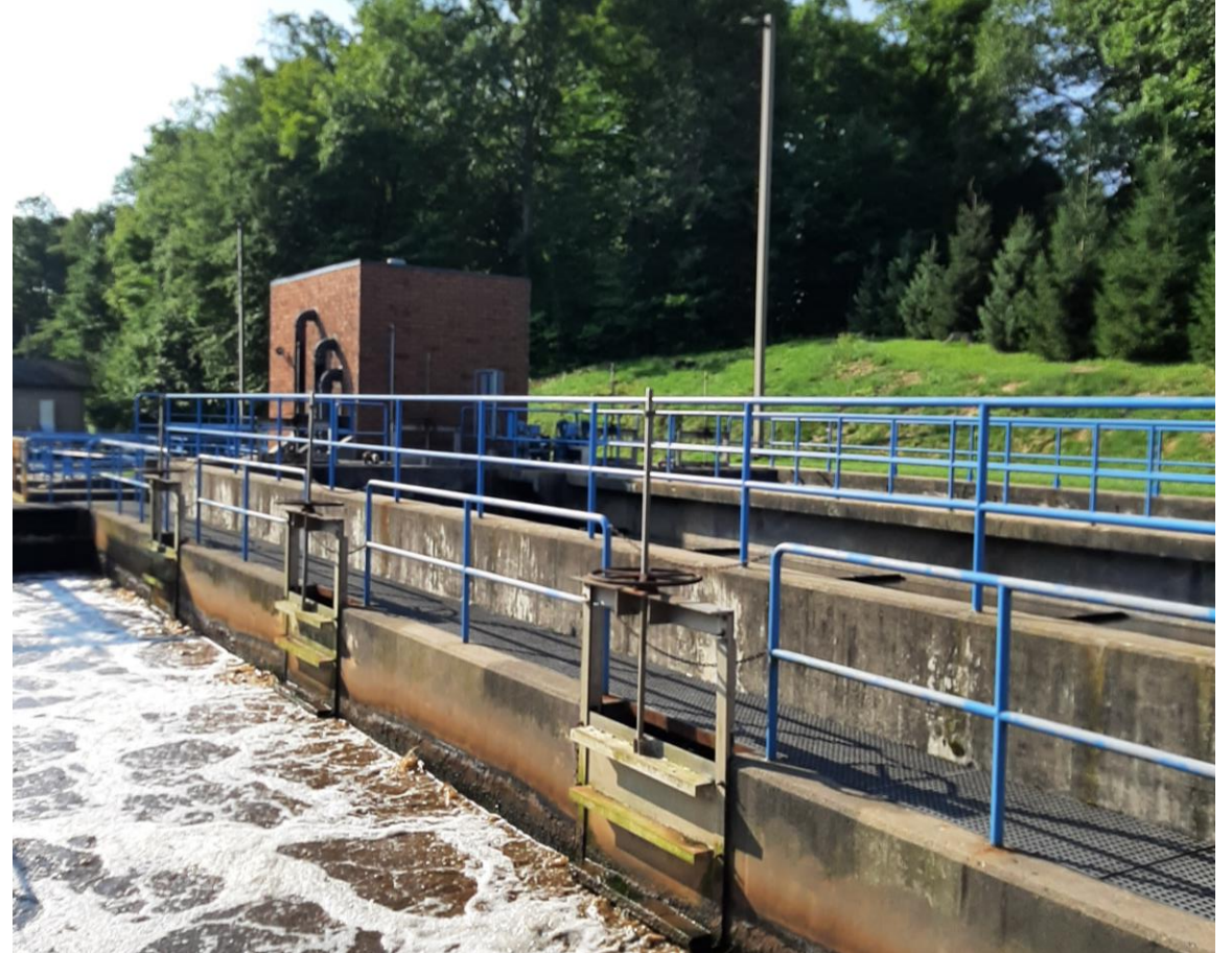
Existing Aeration Tanks
