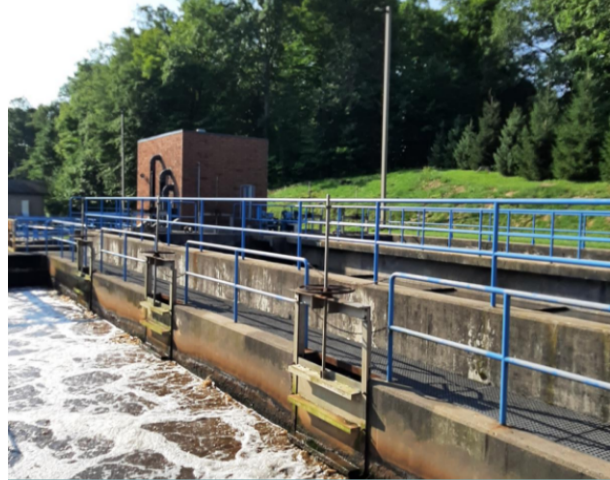
Existing Aeration Tanks
